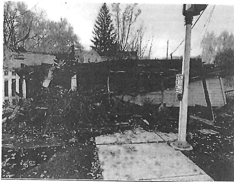
Remaining House Structure, 10/22/2020 Looking South
