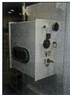
Figure 7. External visible break with gauges.
