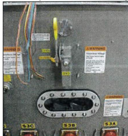
Figure 8. VFI transformer with visible break.
